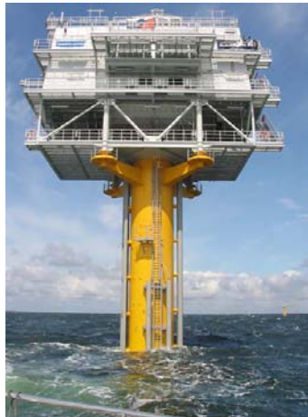
140 MVA, 145 kV offshore substation in the Netherlands
